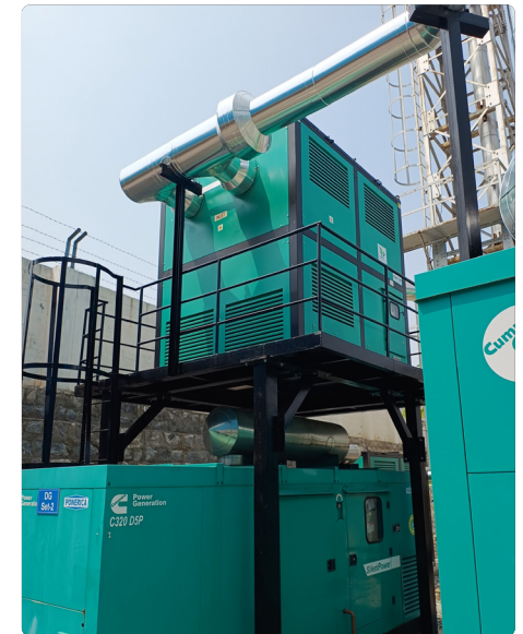
RECD installed at Ather factory.
