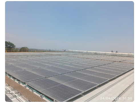
Solar panels on the roof of the Ather factory.
